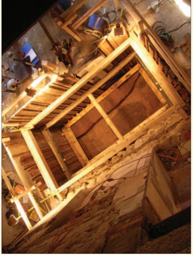
Fig. 15 The excavation of a lift pit at Jesus College in 2008 shows the depth of archaeological deposits in the city centre. The dark amorphous shape at its base is a rubbish pit cut into the natural gravel. To the right are a line of stake holes representing the remains of a Late Saxon building fronting onto Market Street.
